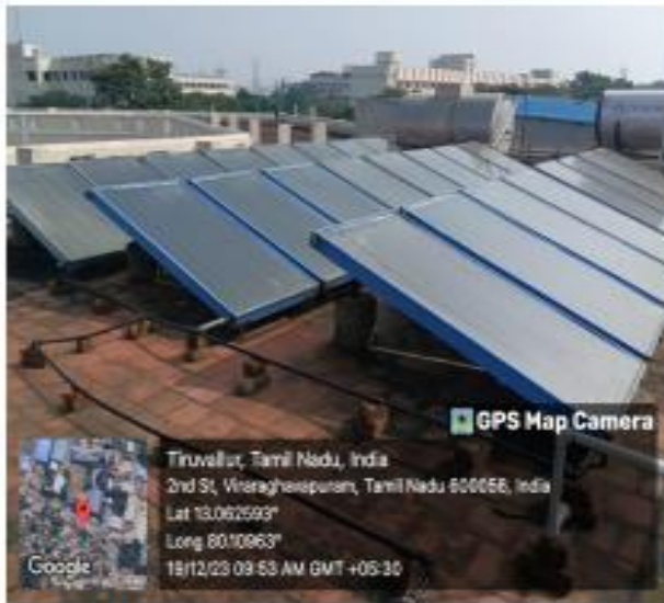
SOLAR WATER HEATERS
